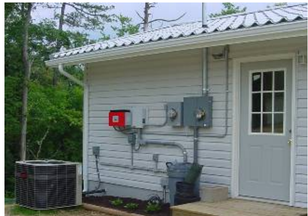
Figure 48. Sunny Boy (red box at left) installed in TVA-approved Green Power
