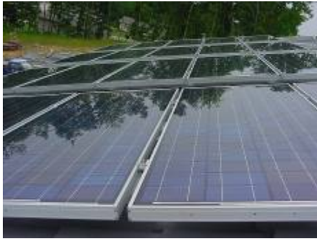
Figure 46. Modules are clamped to aluminum rails and carefully grounded.
