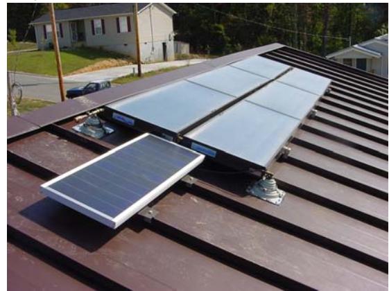
Figure 7. Solar Water Heater collectors.
