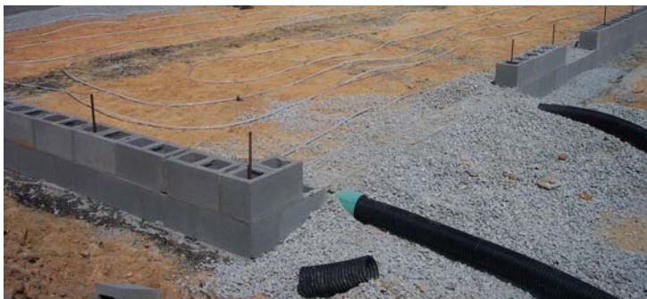
Figure 25. Footer drains run to daylight on both sides of the wall below the basement floor.
