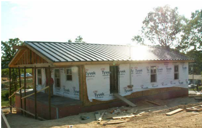
Figure 30. Infrared selective coating was used on the brown raised metal roof to cover ZEH5.
