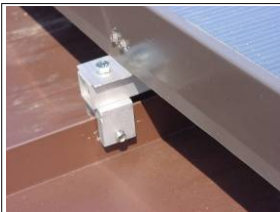
Figure 31. S-5 mini clip holding a solar module on ZEH5 to the raised metal seam.
